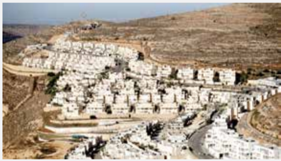
A general view shows construction of the illegal Israeli settlement of Ramat Givat Zeev in the occupied West Bank. REUTERS
