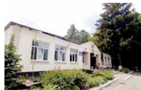
↑ This image taken from a video shows a damaged building in the Belgorod region, Russia, on May 22, 2023. ● AP
