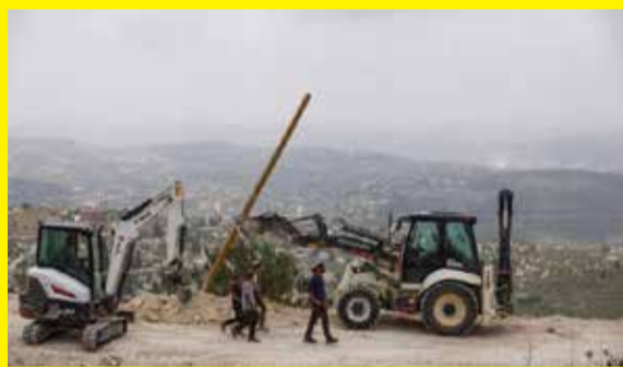
◀ Israeli settlers walk past construction machinery after structures were erected for a new Jewish seminary school in the settler outpost of Homesh in the Israeli-occupied West Bank, on May 29, 2023. ● RONEN ZVULUM/REUTERS
