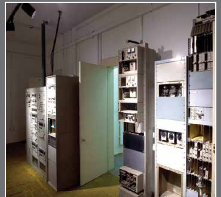
The devices on the right are remains of electronic equipment. On the left, there is a satellite device for sending and receiving information, which is connected to a satellite antenna.
