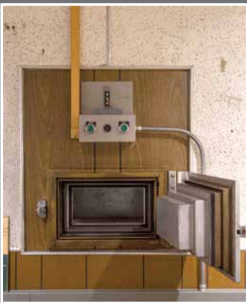
Communications door to the other section of the container.
