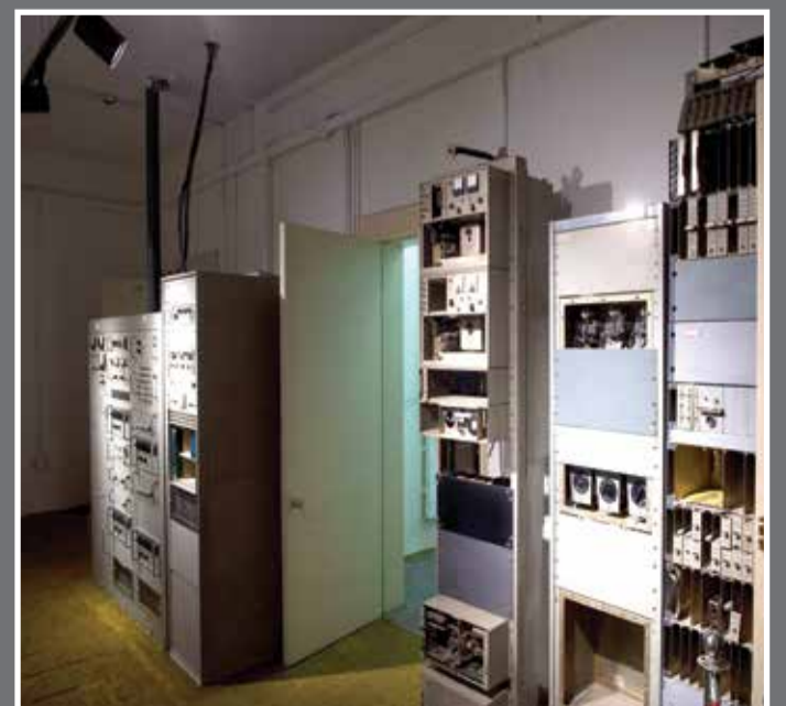
The devices on the right are remains of electronic equipment. On the left, there is a satellite device for sending and receiving information, which is connected to a satellite antenna.
