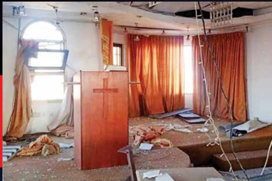
Damage at Gaza Baptist Church after a blast on December 26, 2023 ● RAMABDU/X
