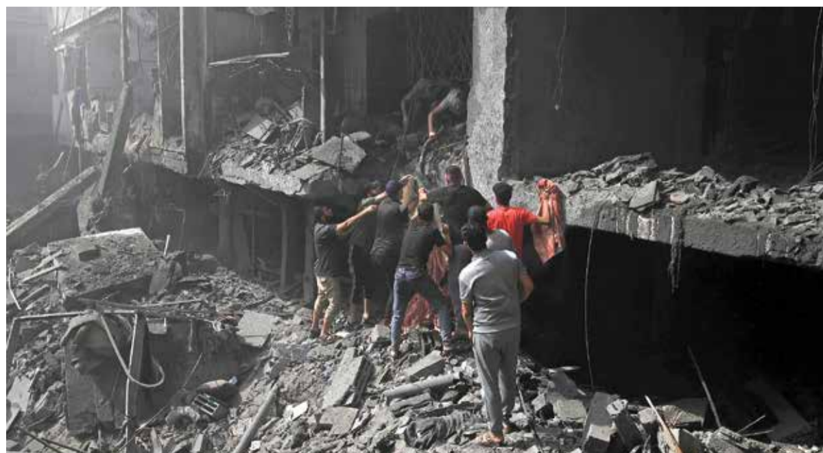
Palestinians try to rescue survivors and pull bodies from the rubble after Israeli air strikes hit buildings near Al-Aqsa Martyrs Hospital in Deir al-Balah, central Gaza, on October 22, 2023.
