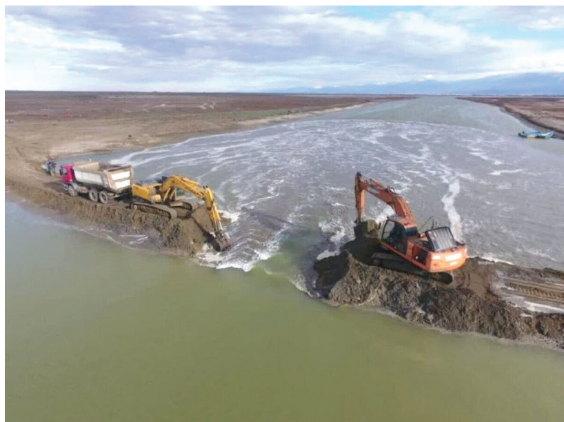
Heavy machinery work to open the Ashuradeh Canal in 2023, allowing water to flow from the Caspian Sea into the drying Gorgan Bay. ● BORNA
