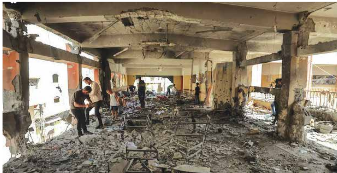
Palestinians inspect the damage to a school sheltering displaced people after it was hit by an Israeli strike, amid the Israeli war on Gaza, at Beach refugee camp in Gaza City, on September 22, 2024.
