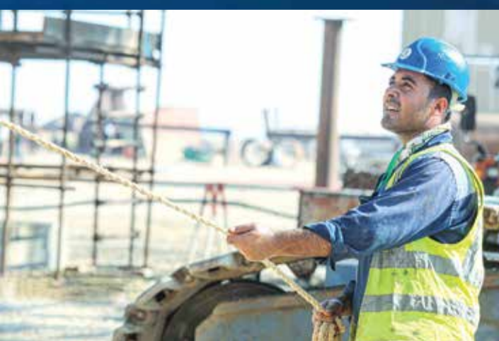
An engineer at work on the jacket installation of the A platform of Phase 11 of the South Pars gas field on August 16, 2024. The jacket of the A platform of Phase 11, weighing around 4000 tons and 77 meters high, is one of the largest marine structures in the country, whose construction began in June 2024 and will be transferred to its location in the South Pars common gas field in the Persian Gulf in the coming months.
