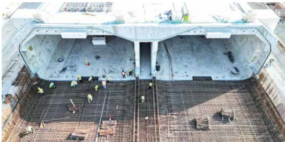
Workers are constructing the tunnel that will connect Iraq's coastal region to international trade links through Turkey, in al-Faw, Iraq, on February 8, 2024. ● MOHAMMED ATY/REUTERS
