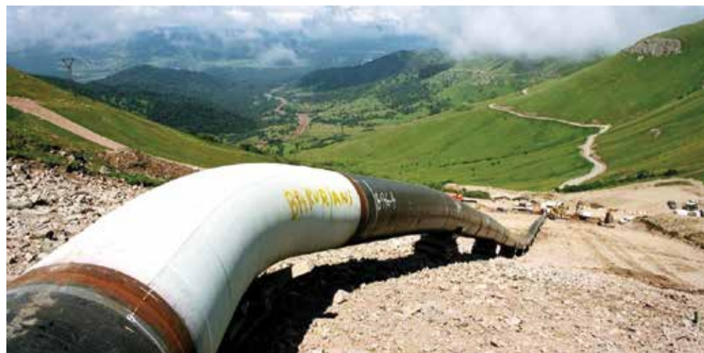
Baku-Tbilisi-Ceyhan pipeline ● minenergy.gov.az
