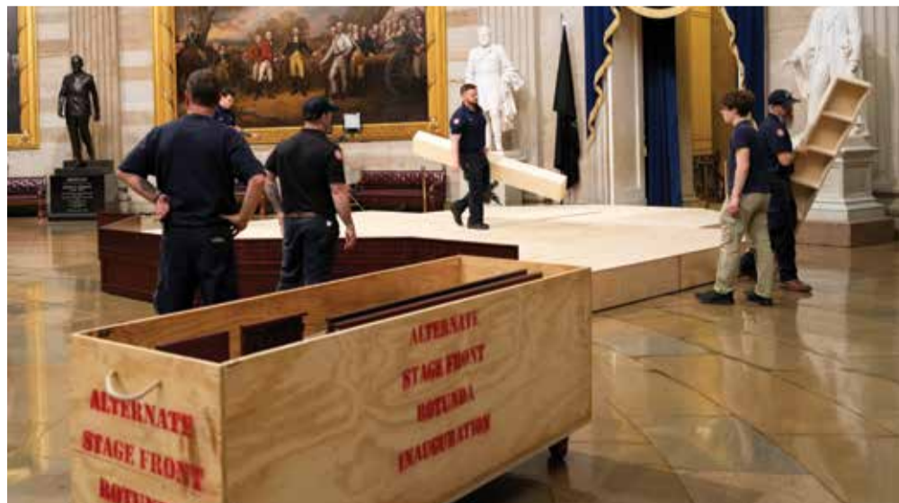
Workers build a stage in the US Capitol Rotunda in Washington on January 17, 2025, for the 60th presidential inauguration, which was moved indoors.
