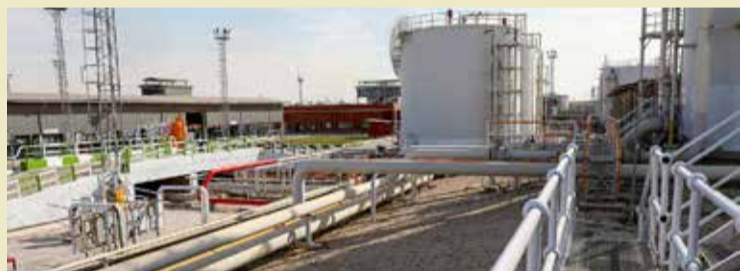
The photo shows Iran's largest oil desalination plant in Ahvaz, southwestern Iran, which was inaugurated remotely by President Masoud Pezeshkian on January 22, 2025.
