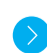
The jacket for the Belal Gas Field development project, constructed with a $16 million investment, is loaded out from the Sadra Yard in Bushehr, southern Iran, on January 22, 2025. ● ALIREZA KHAZRAEI/SHANA
