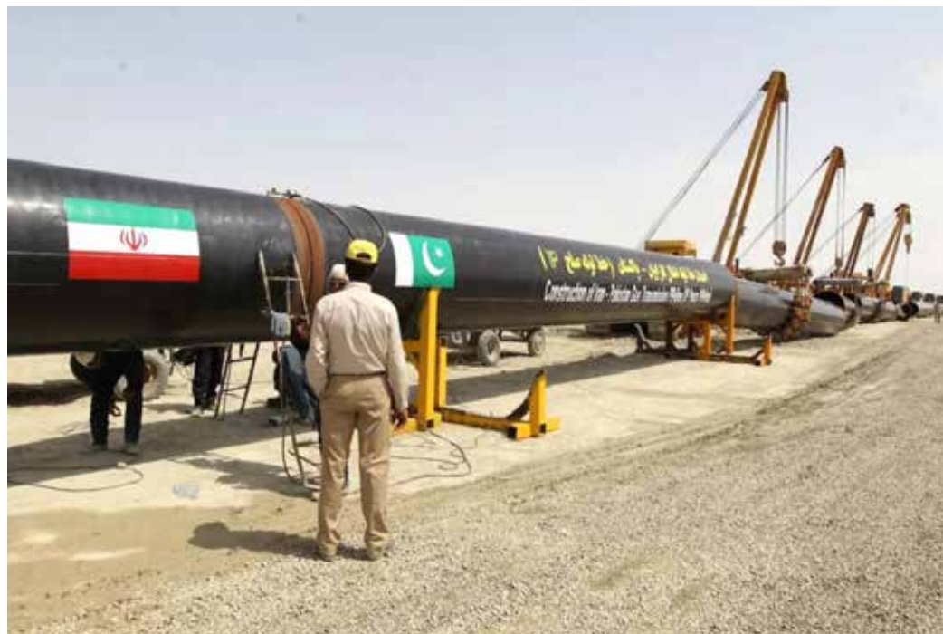
Iranians work on a section of a pipeline linking Iran and Pakistan near the Iranian port city of Chabahar on March 11, 2013. ● ATTA KENARE/AFP
