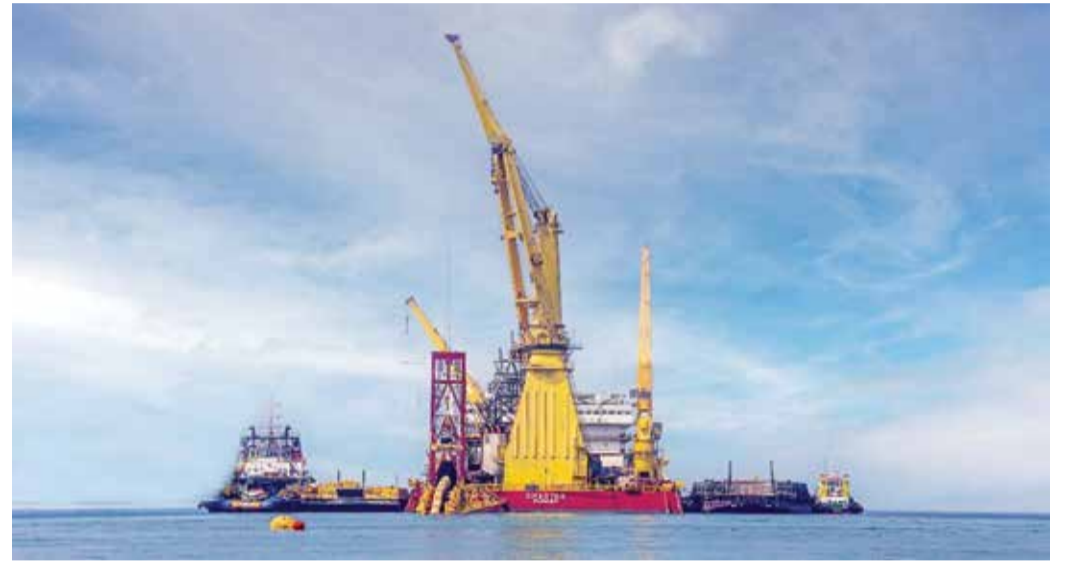
The initial phase of the new pipeline project in South Pars Phase 16 reaches completion. ● ALI SOLEIMANI/SHANA
