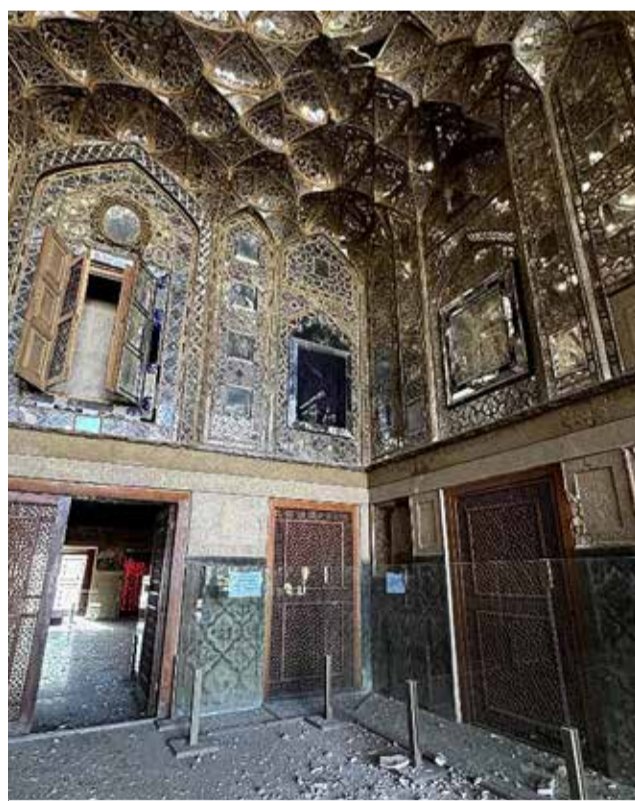
The photo shows the damage done to the windows and fittings of the Chehel Sotoun Palace in Isfahan. ● IRNA
