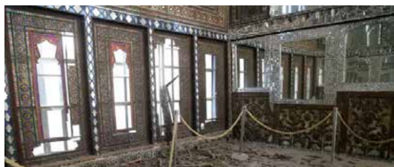
Broken glass and decorative fragments cover the floor of a mirror hall inside the Golestan Palace in Tehran after nearby explosions damaged the historic complex in Tehran, following recent American-Israeli strikes on Iran, in March 2026.
