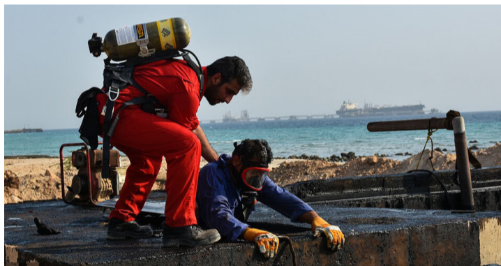
The file photo shows workers fixing a crude oil leak from a pipeline on Kharg Island on August 7, 2025.
