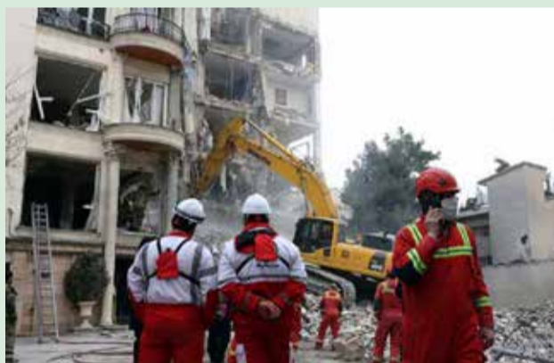
Iranian firefighters with the help of an excavator clear rubble from a destroyed residential building in northern Tehran. ● IRNA
