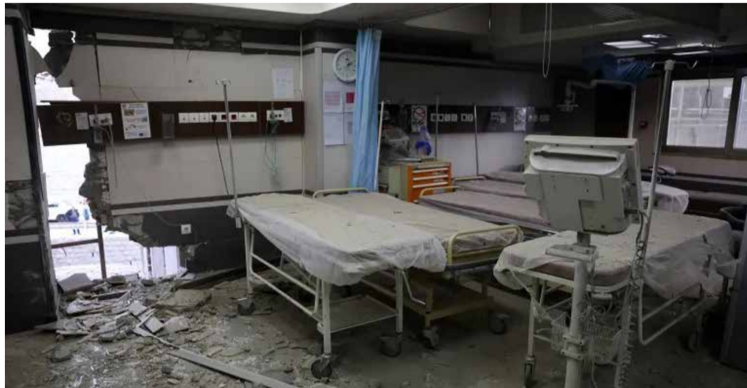
A room in Gandhi Hospital in Tehran, Iran, is damaged and subsequently evacuated as a result of US-Israeli air strikes on March 1, 2026. ● ABEDIN TAHERKENAREH/EPA
