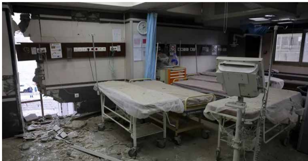
A room in Gandhi Hospital in Tehran, Iran, is damaged and subsequently evacuated as a result of US-Israeli air strikes on March 1, 2026. ● ABEDIN TAHERKENAREH/EPA
