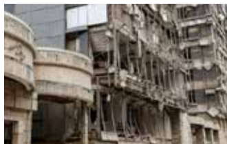
Extensive damage to Gandhi Hospital in northern Tehran following US-Israeli airstrikes on early March 2026. ● IRNA
