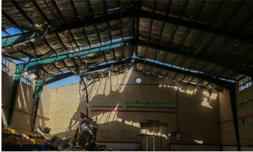
The photo shows a damaged sports hall in Lamerd, southern Iran, that was attacked by the US and Israel on February 28, 2026, while a women's volleyball team was using the facility.
