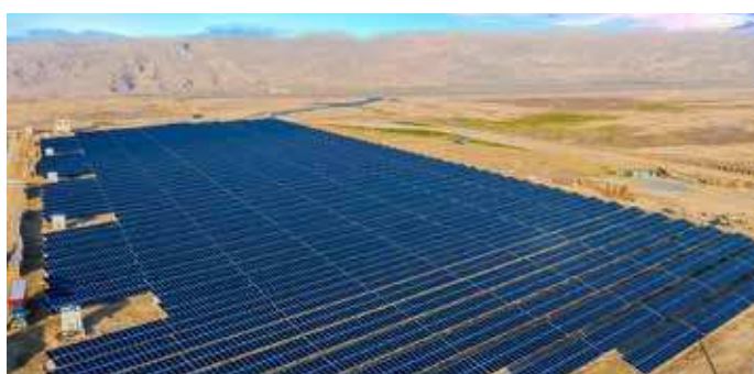
A large solar farm has been constructed in the Lamerd Special Economic Zone. ● lamerdsez.ir
