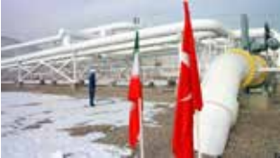
A section of the Iran-Turkey natural gas pipeline is seen near the border between the two countries.
